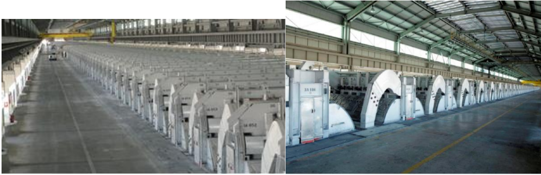
Figure 6. DX (left) [6] and DX+ (right) [7] potroom in Al Taweelah.
